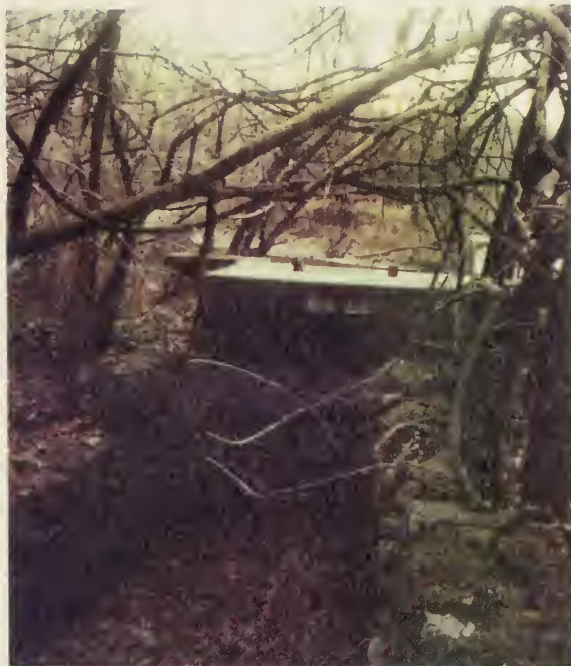
Fig. 114 Masonry sluice gate for one of the races at Snyder's Mill near its juncture with the French Creek. Photograph by the author, 1994.
